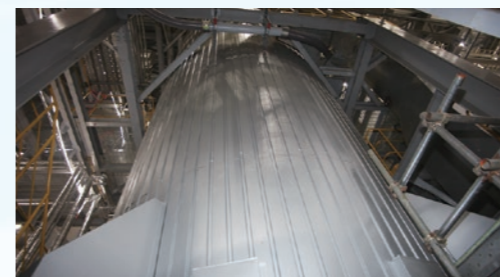
減温塔 Cooling tower
