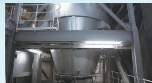
飛灰貯留槽 Fly ash storage tank
